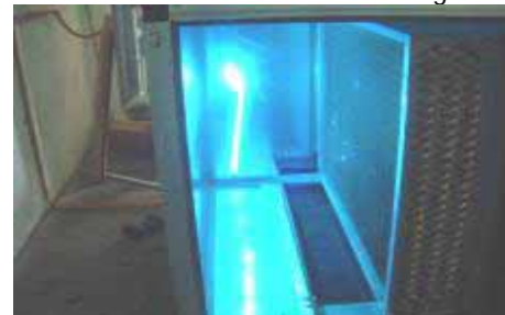
Emitters installed behind the cooling coil
