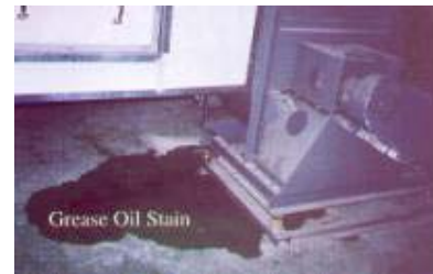
Typical oil drip and leak from ducts
